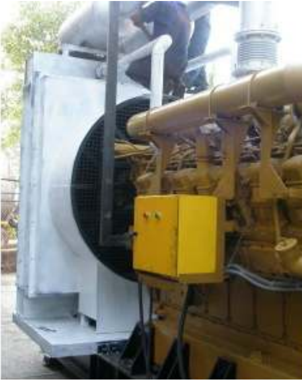
Radiators with Fan Mounted Direct on Motor
